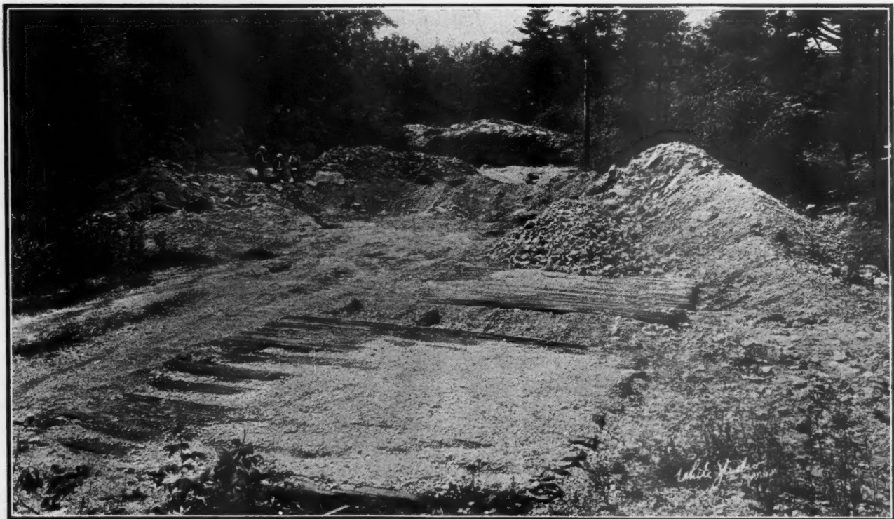
Entrance to Pit Number One. Face is About 100 Feet Wide and 35 Feet High
